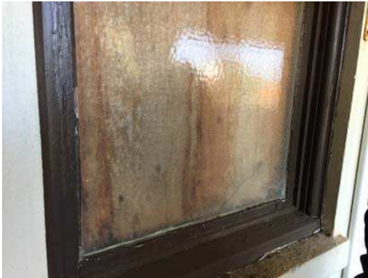
Photo #9: Atherton building. Wood windows with asbestos containing caulking.
