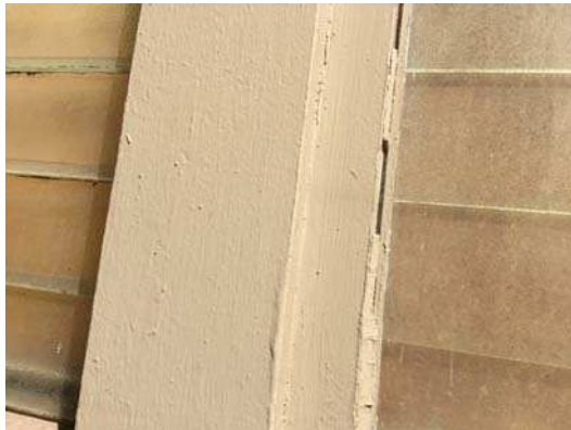
Photo #12: Atherton building. Wood windows with asbestos containing glazing (interior of the frame).
