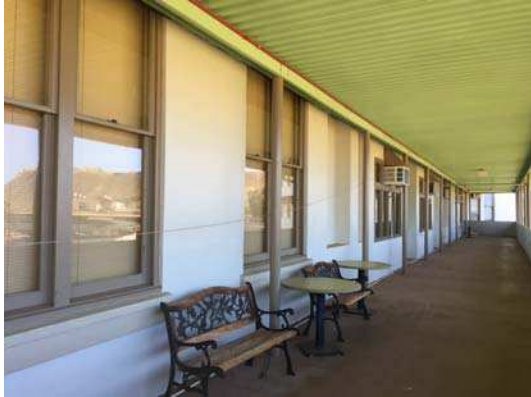
Photo #13: Administration building. Wood windows with asbestos containing caulking and glazing (interior of the frame).
