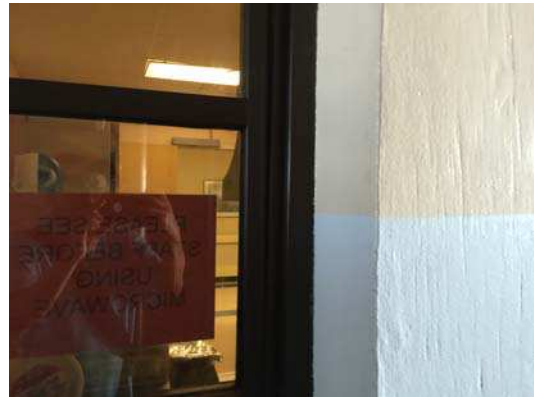
Photo #2: Young building. Metal windows with asbestos containing caulking.
