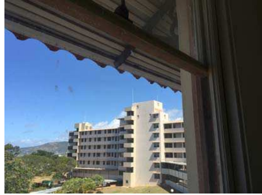
Photo #8: Atherton building. Wood windows with asbestos containing caulking.
