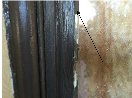
Photo #10: Atherton building. Wood windows with asbestos containing glazing (interior of the frame).
