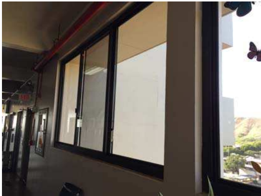
Photo #1: Young building. Metal windows with asbestos containing caulking.
