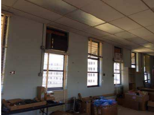
Photo #7: Atherton building. Metal windows with asbestos containing caulking.
