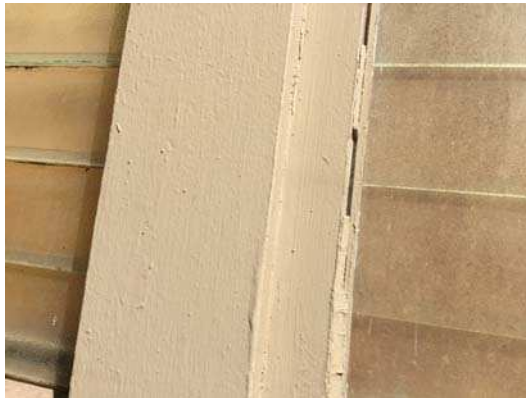
Photo #12: Atherton building. Wood windows with asbestos containing glazing (interior of the frame).
