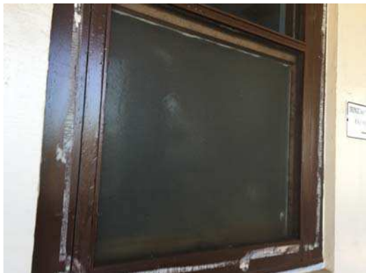
Photo #6: Young building. Wood windows with asbestos containing caulking.
