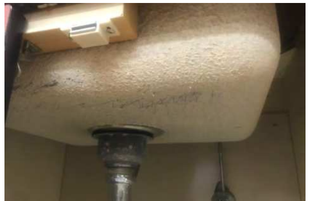
Photo 12: Beige sink undercoat. Non-ACM.
