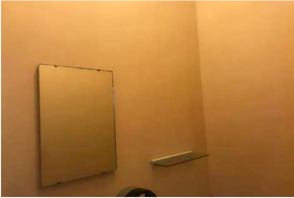
Photo 7P: UCERA's toilet drywall partitions. Tan paint with lead.
