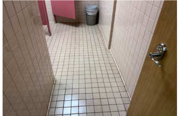
Photo 8: 4"x4" tan ceramic floor tile with brown grout and gray mortar. Non-ACM.
